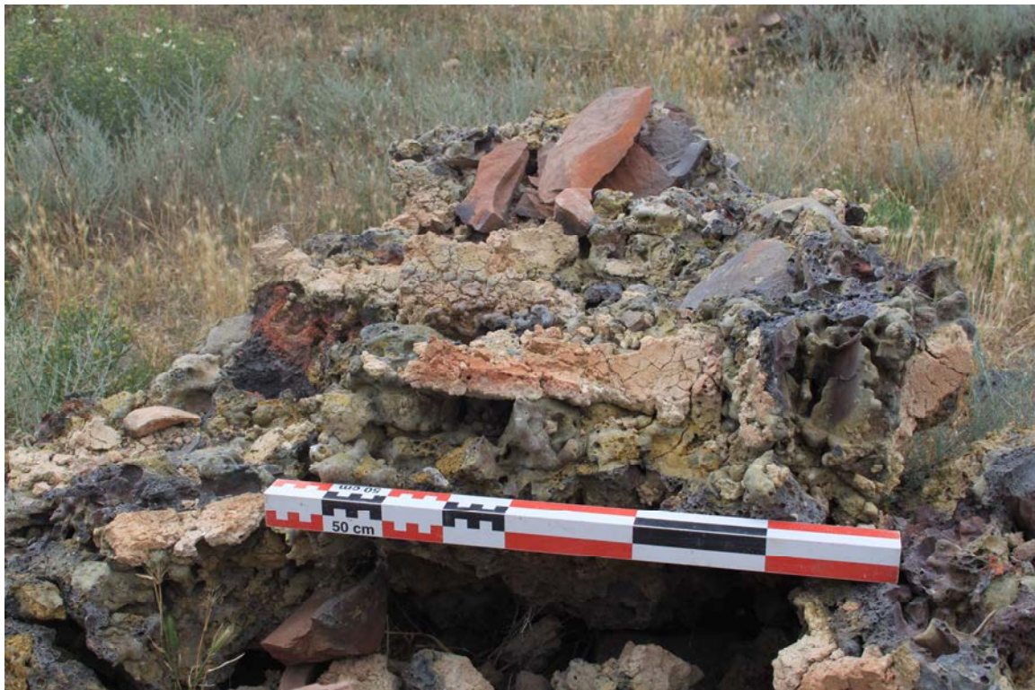
Fig. 28. Detail of one of the walls, showing the main degradation phenomena affecting the building.
